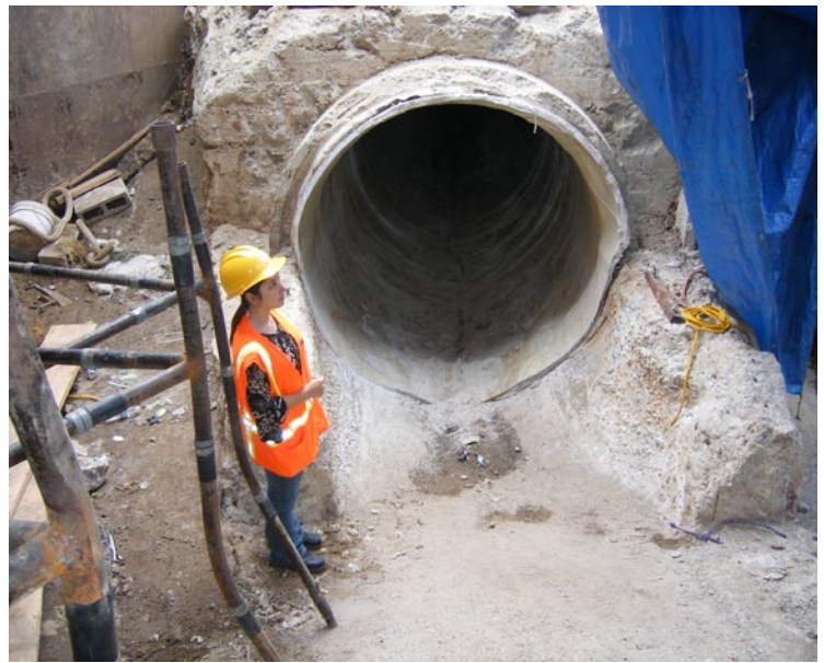
CIPP lined siphon inlet.
